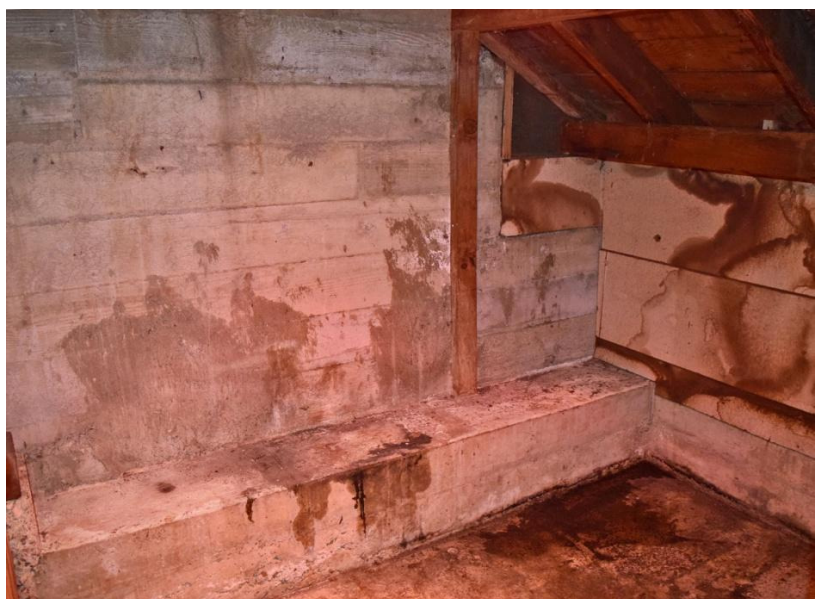
The south side of the Beer Room, showing the concrete footing from where I launched a significant quantity of my Dad's beer to the floor.
